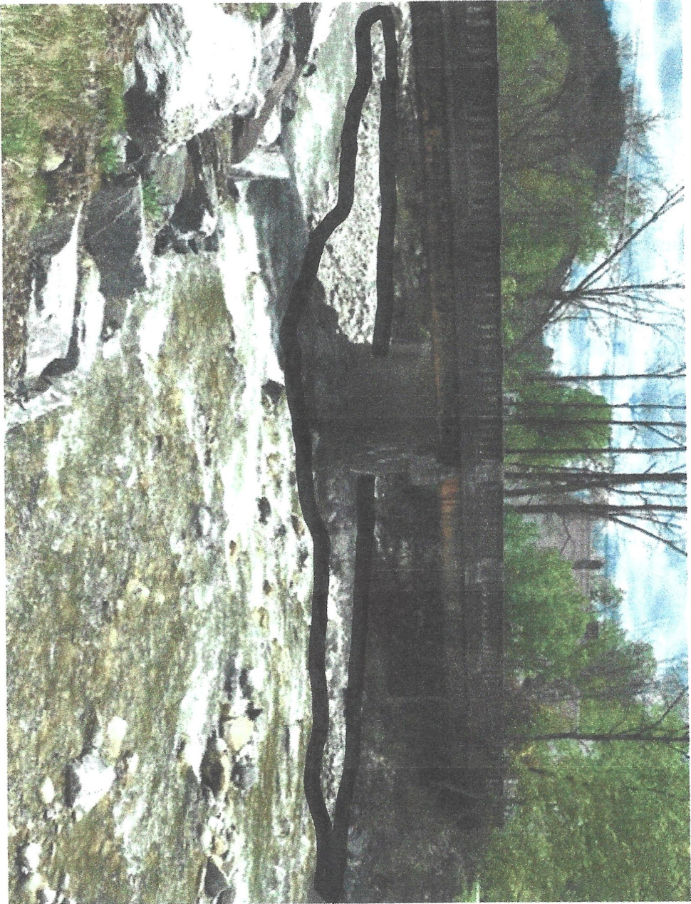
Site B - Under Depot Street Bridge - Deposition
